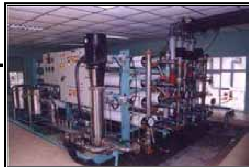
CSMCRI's 1 MLD Plant installed in November 2003
